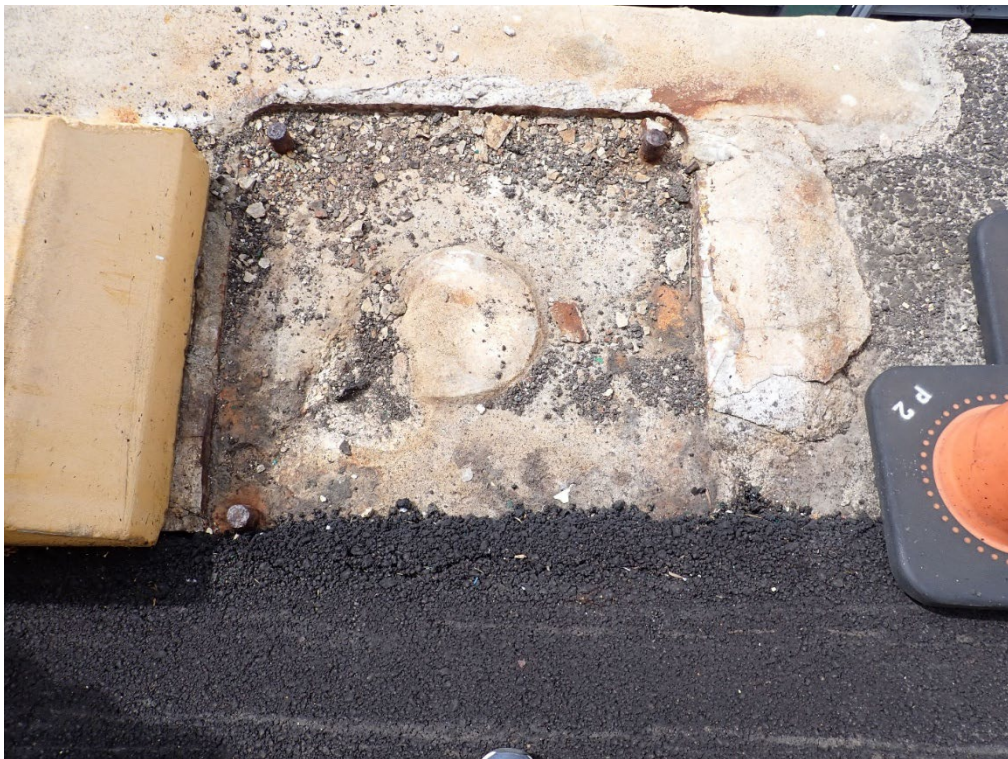
Photo 2: Missing Type A2 Bollard
